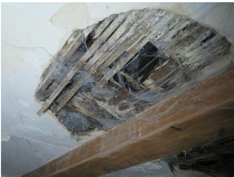
Photo 9- Guano covered timbers above collapsed ground floor ceiling
