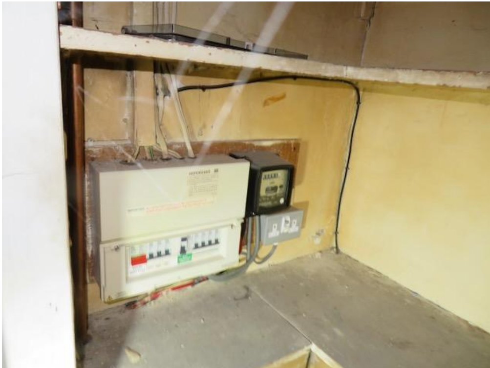
Photo 14 – Electrical meter and consumer unit.
