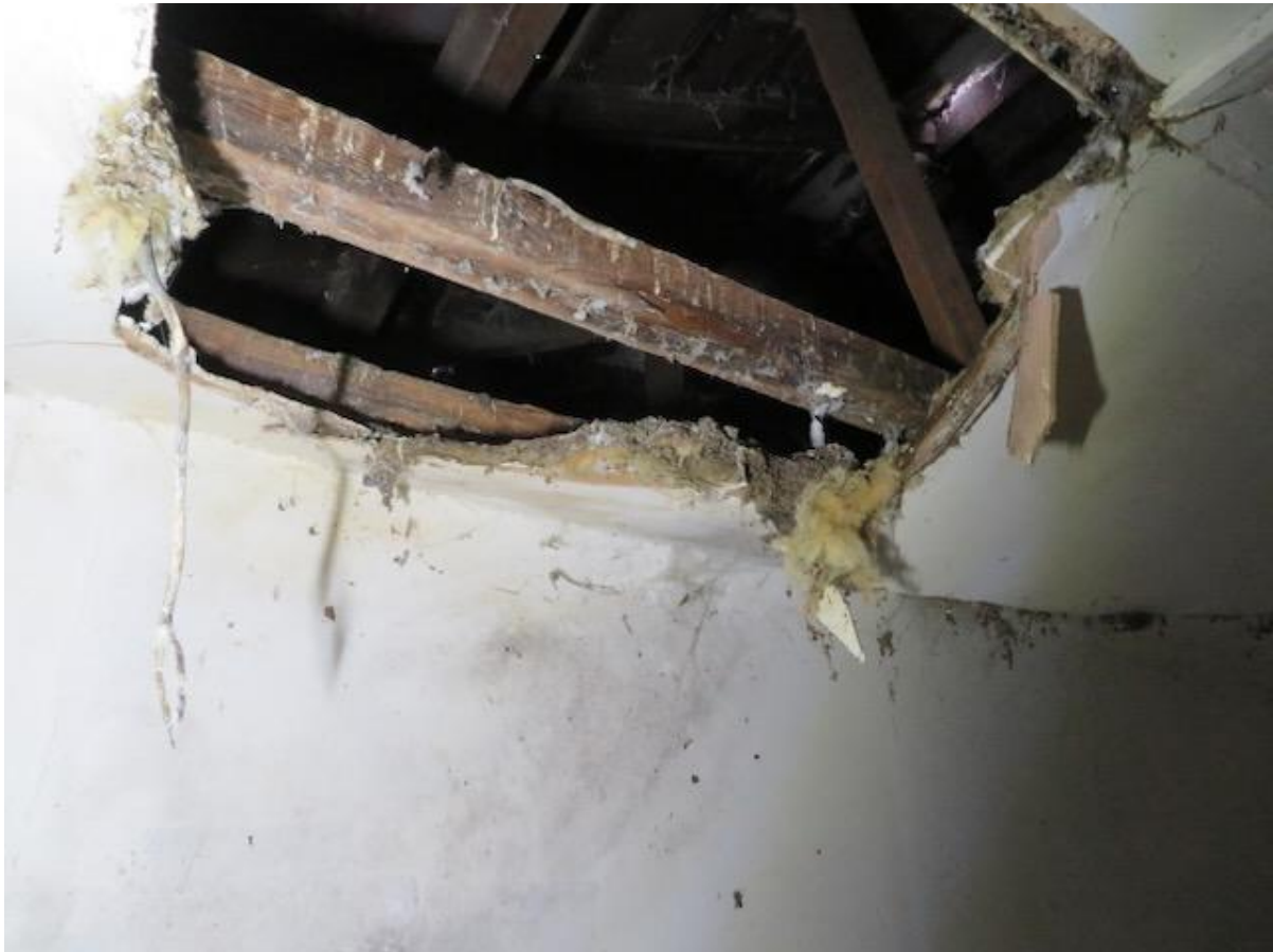
Photo 5- Collapsed first floor ceiling
