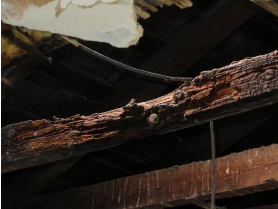
Photo 8- Rotted through roof tie
