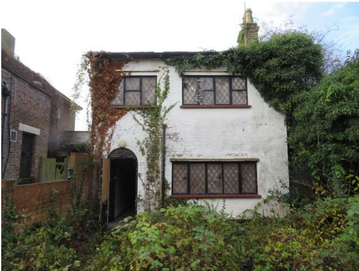
Photo 1- Front Elevation – Overgrown External walls
