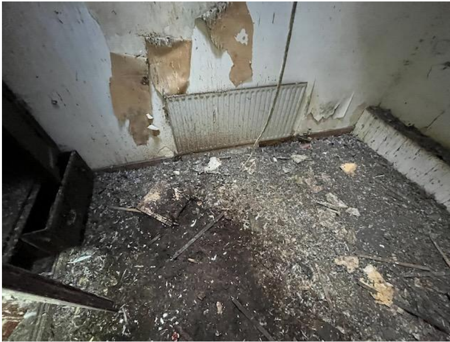
Photo 10- Guano covered first floor finishes
