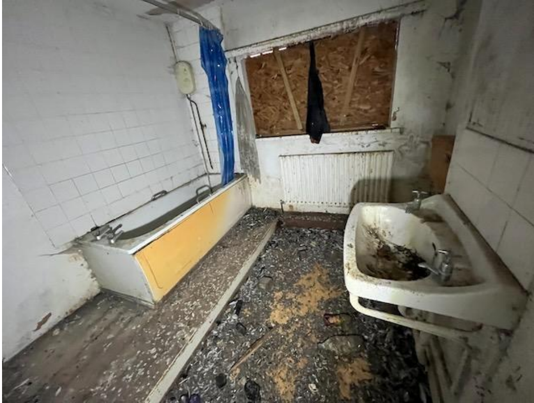
Photo 15- Guano covered bathroom fittings
