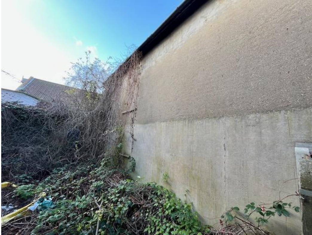
Photo 3 - Cracked render overgrown with shrubs
