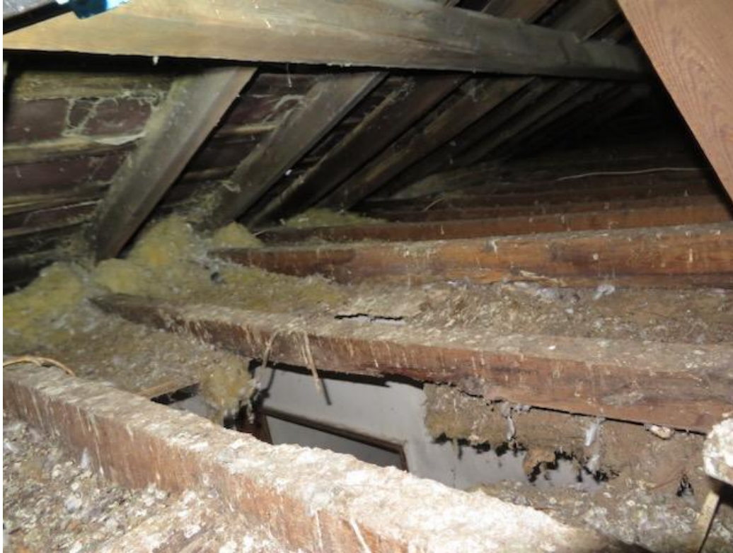
Photo 6- Guano covered timbers above collapsed first floor ceiling
